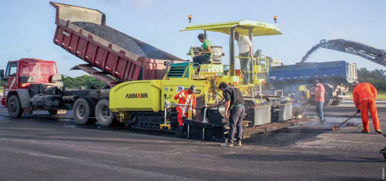
Parts of the apron were refurbished and resurfaced with asphalt during one of the first phases of the project. The demands placed on the quality of the asphalt laid at the airport are especially high, but nonetheless easily achievable with the Ammann AFT 500 G.
