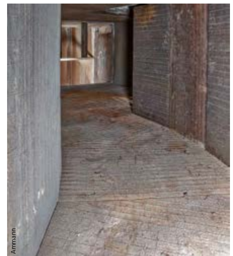
A crude gas channel on an asphalt mixing plant clad in Amdurit plates.
