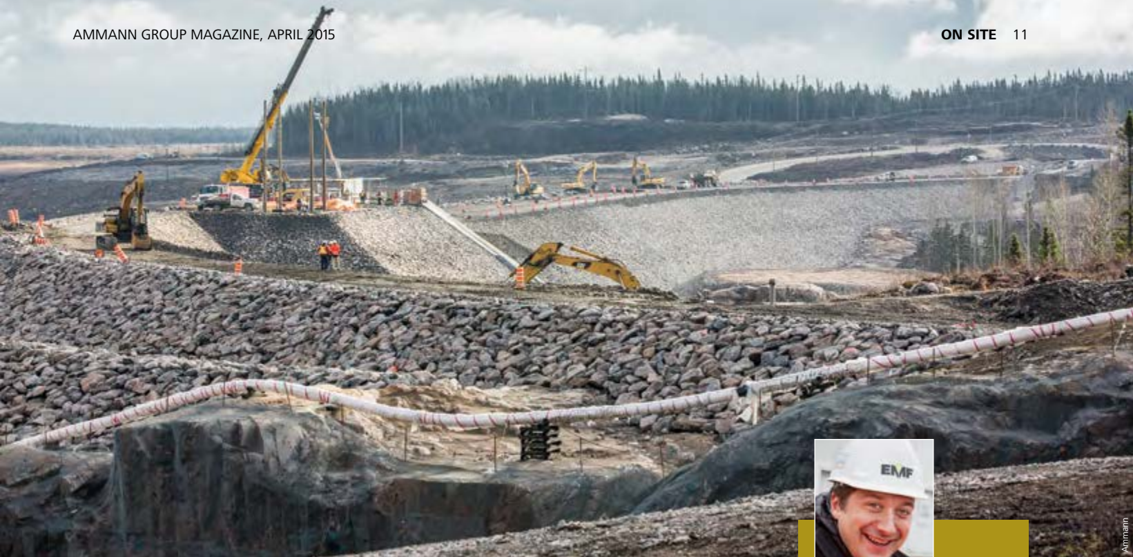
At 40 metres high and 830 metres long, the Romaine 1 dam is a structure of huge proportions.
