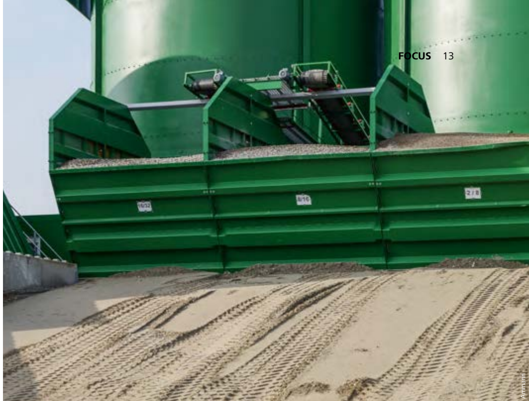
Whilst chambers 1 and 2 of the feed bins are loaded directly via conveyors, wheel loaders are used for the other chambers.
